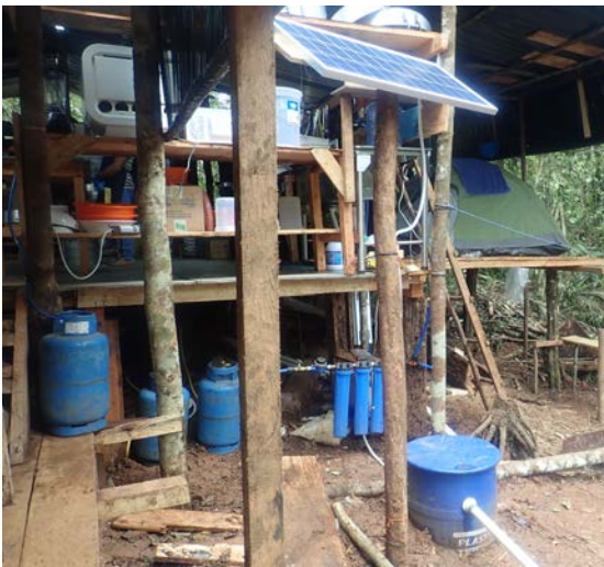
Figure 6. Stream water is filtered for potability
