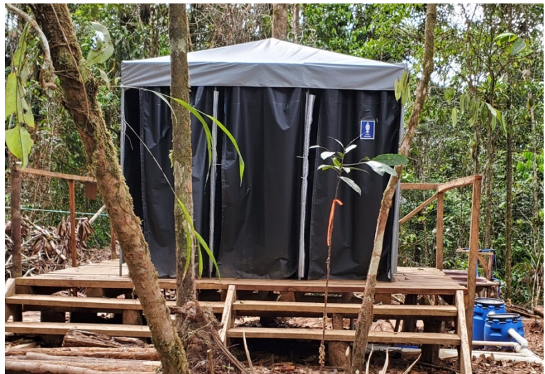
Figure 4. Latrine at a drill camp. Water from the latrines drains into a biodigester where the sewage is broken down organically.
